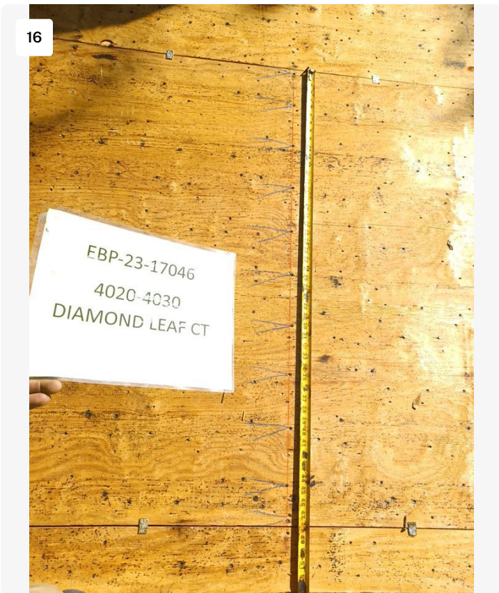
Project: 4030 Diamond Leaf Ct Date: 10/24/2023, 11:50am Creator: Lucio Roofer
