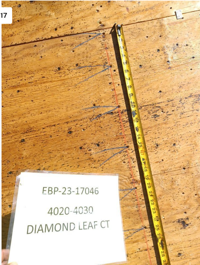
Project: 4030 Diamond Leaf Ct Date: 10/24/2023, 11:50am Creator: Lucio Roofer
