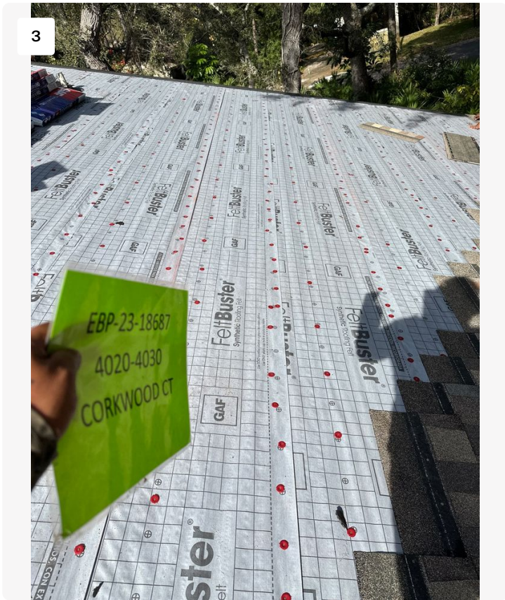
Project: STRATHMORE GATE - 4020-4030 CORKWOOD CT / 2310-5005564-01 Date: 1/17/2024, 1:32pm Creator: Maynor Perez
